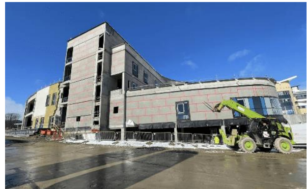
Baird south east elevation facing Westburn Road – cement particle board (CPB) installed, sealed and taped (red squares) in preparation for insulation followed by render.
