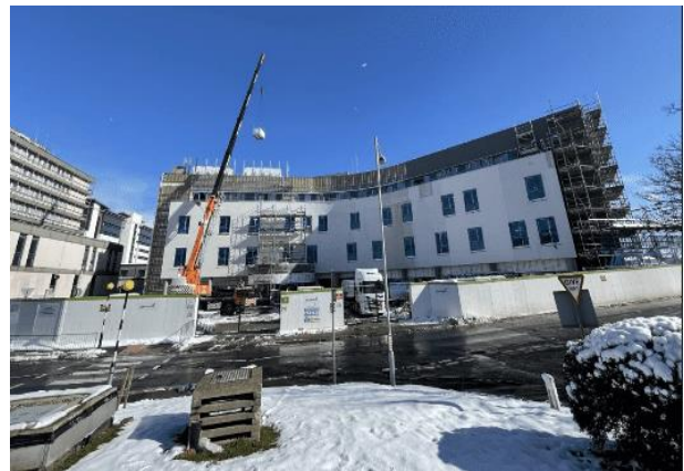
Baird west elevation (main entrance) facing Foresterhill Road – second/final coat render ongoing. Notice also the crane in action lifting an air handling unit into place on the rooftop plantroom.
