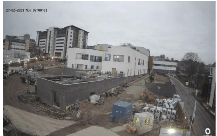
The ANCHOR Centre south elevation - ongoing road formation, landscaping and groundworks to the south and east of the site.
