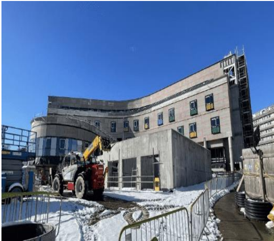
Baird east elevation – cement particle board nearly complete, taped and sealed in preparation for insulation followed by render. Concrete Generator Housing in foreground.
