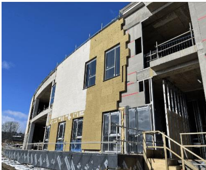
Baird south elevation facing Westburn Road – mineral insulation and scratch coat render is ongoing.
